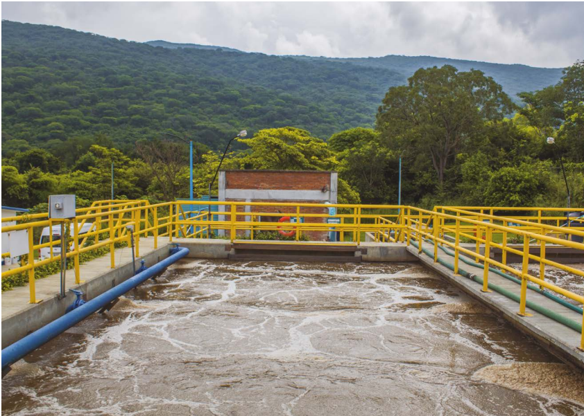
Figure 14. The wastewater treatment plant at Jalpan de Serra. It treats water from the city, not just black and graywater from homes, but also runoff from the streets. In addition, clean water from a spring under the city is directed into the wastewater stream. As a result, the system often exceeds its capacity in terms of volumes of water, particularly during the wet season, and then is not capable to clean the water to a desirable quality before discharge into the Rio Jalpan.
